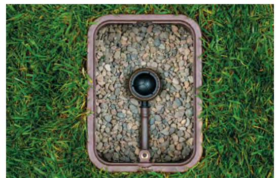
Automatic Flush Valve Installed
