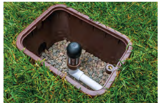
Air/Vacuum Relief Valve Installed
