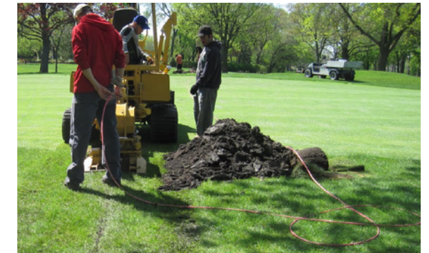
VIBRATORY PLOWS CUT SLOTS IN THE SOIL RATHER THAN DIGGING A TRENCH RESULTING IN VERY LITTLE DAMAGE TO THE TURF
